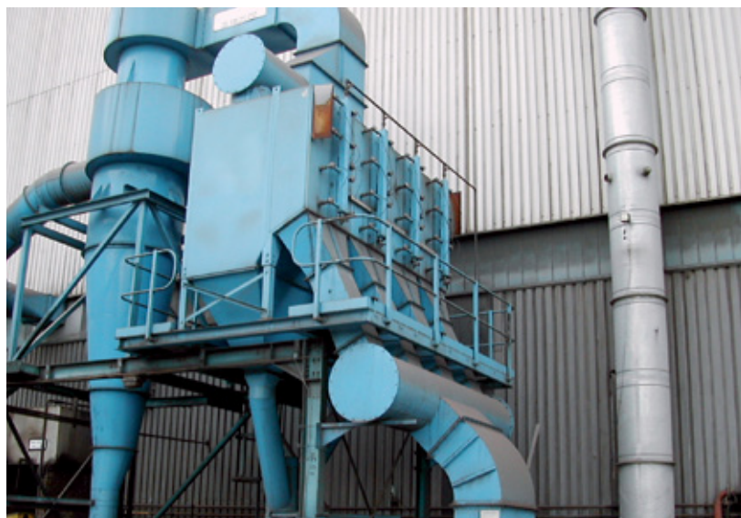
Cartridge filters fitted on rolling mills at stainless steel plant
