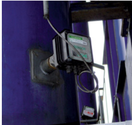
Emissions at hot rolling line monitored by PCME ElectroDynamic™ System
