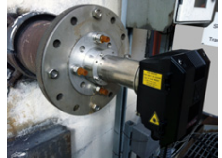
Gas Fired Boiler monitored by ProScatter™ Technology
