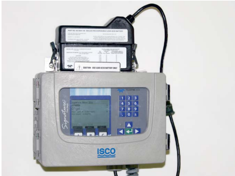
Figure 4-7 Backup battery, installed
