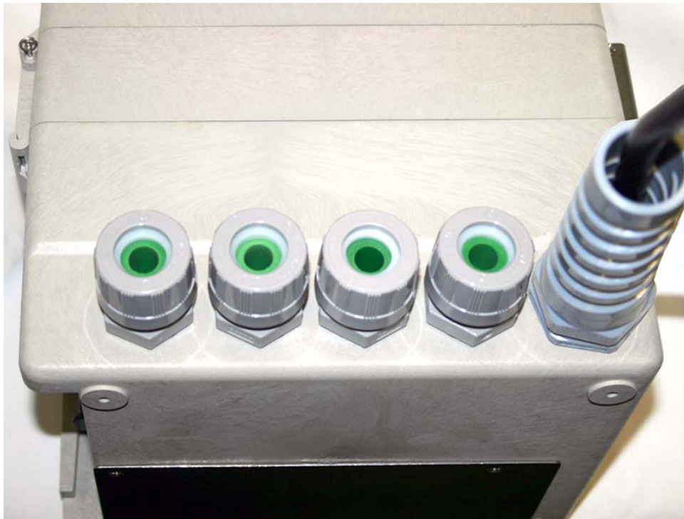
Figure 3-5 Cord-grip fittings installed
