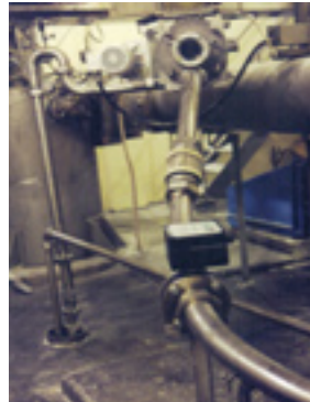
Non-intrusive Flowmasster on 50mm dia Return Fines line
