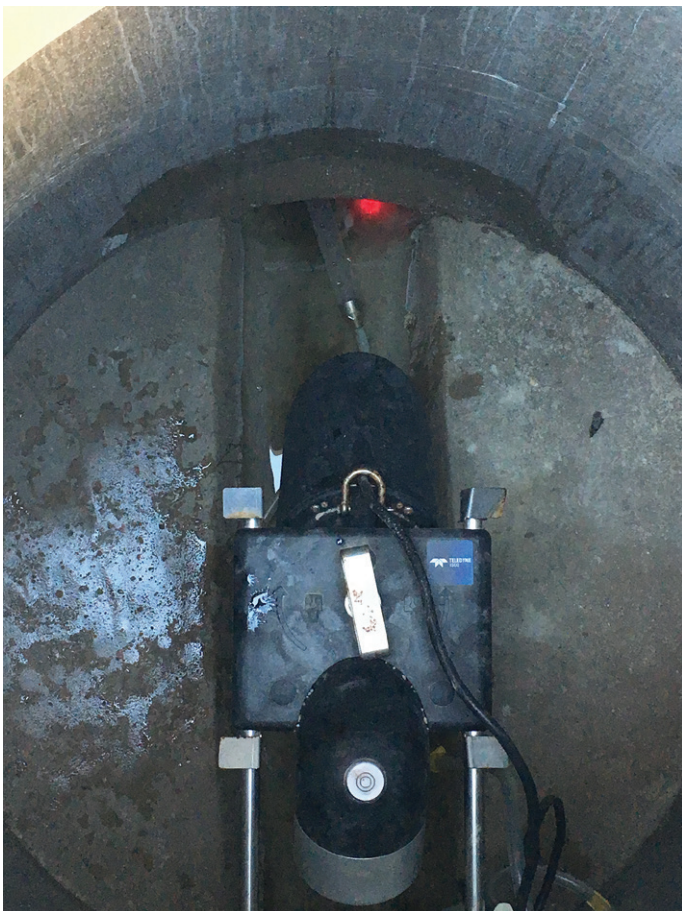
LaserFlow sensor installed in a hospital wastewater effluent.
