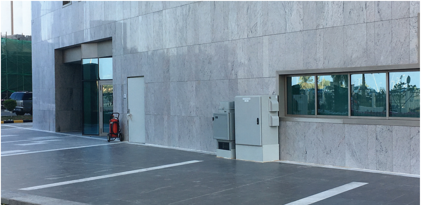
6712FR sampler and Signature flowmeter at Al Amiri Hospital in Kuwait
